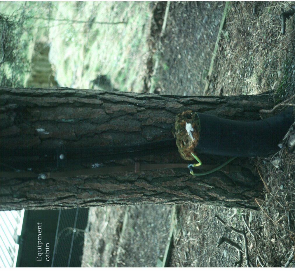
Cables routed under public footpath to equipment cabin 12-15m. away
